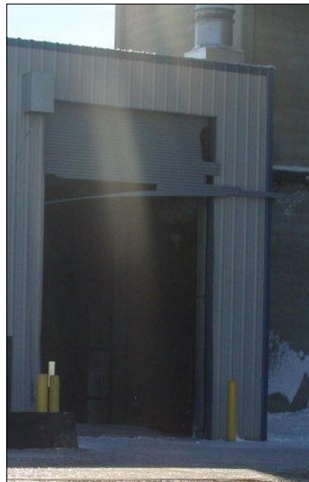
Terminal doors at New Century Ag destroyed by wind.
